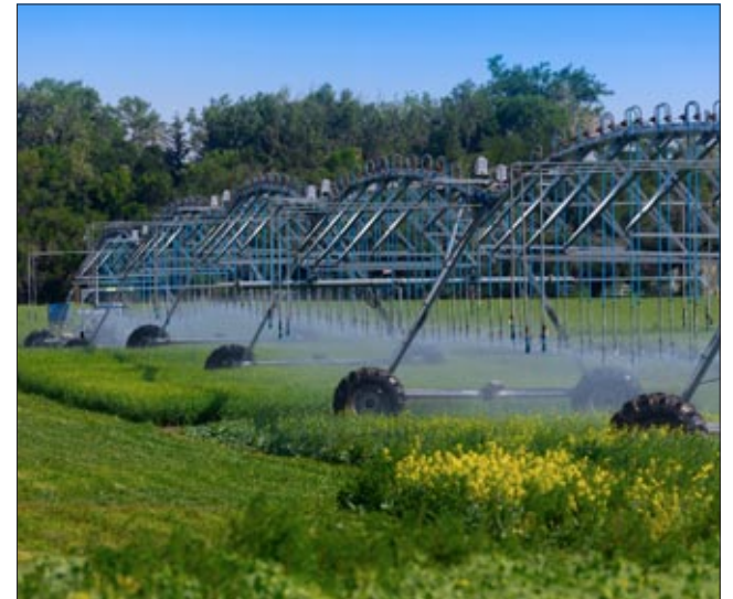
Irrigation infrastructure at the Lethbridge College research farm.
